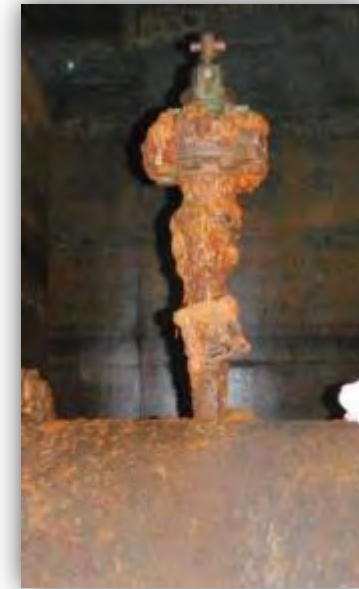
Air valve at Shaft 9A
