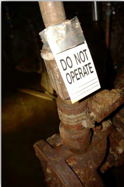
Shaft 8 PRV Chamber
